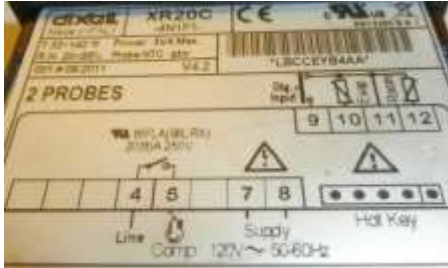
Refrigerator Controller Terminals
