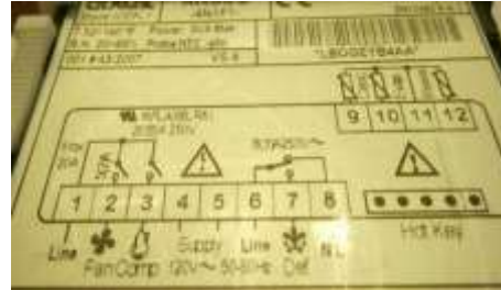
Freezer Controller Terminals
